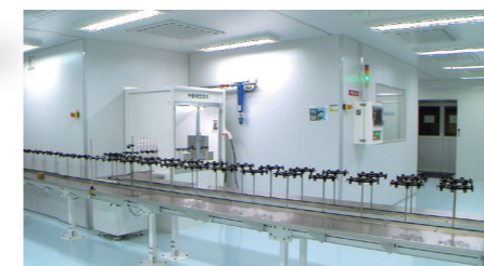
Clean room photo for reference
